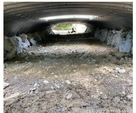
Below Photo - 2722 Stream section built through road crossing to ensure stream function and stability as well as maintaining aquatic organism passage.
