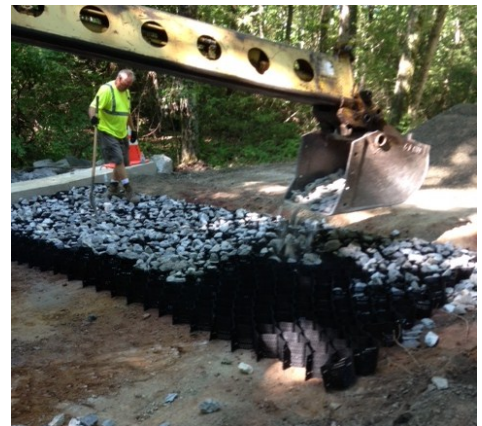
Placement of stone subbase in geotextile web designed to hold road bed in place. Photo courtesy of Polk Township
