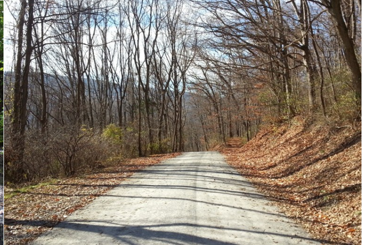
After: Completed crowned road section with paver placed, roller-compacted Driving Surface Aggregate sends runoff to the sides of the road so surface material is not lost.
