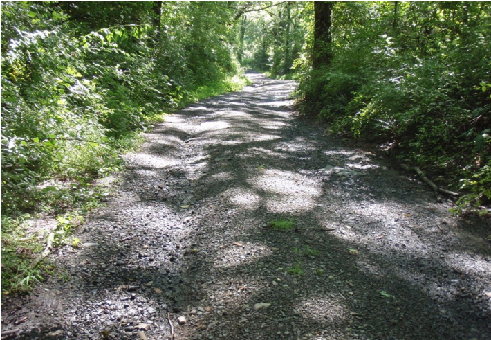
Before: The project runoff was channelized in wheel ruts and road surface material was washing off the road, clogging pipes, ditches, and costing the township money to replace.
